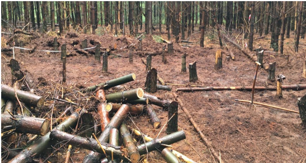
Figure 12 Experimental plots Pst. From top to bottom: Pst before clearing, after clearing, after treatment implementation.
