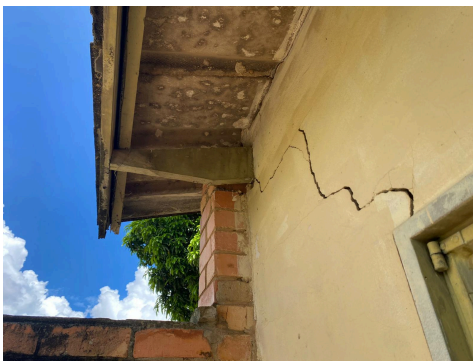
Fig.6 Cracks in a house near the mine.
