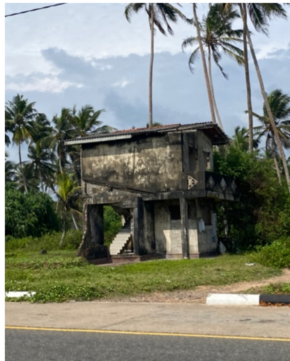
Figure 10. An abandoned house, damaged heavily by the tsunami. Many of such abandoned houses can still be found around Galle.
