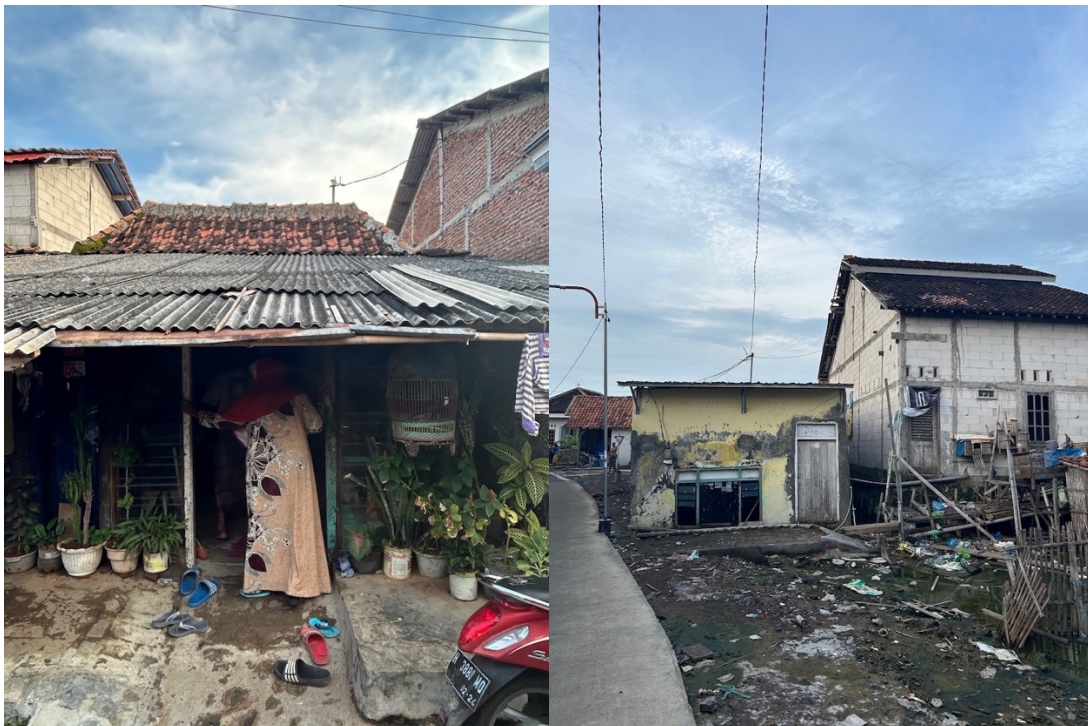
Sinking of houses due to land subsidence. Source: personal archive (April 2024).
