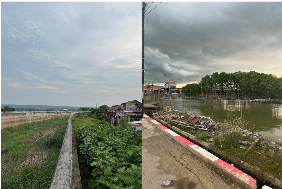
Normalization of the Bringin River (left) and a small wall next to fishponds (right), source: personal archive (April, 2024).
