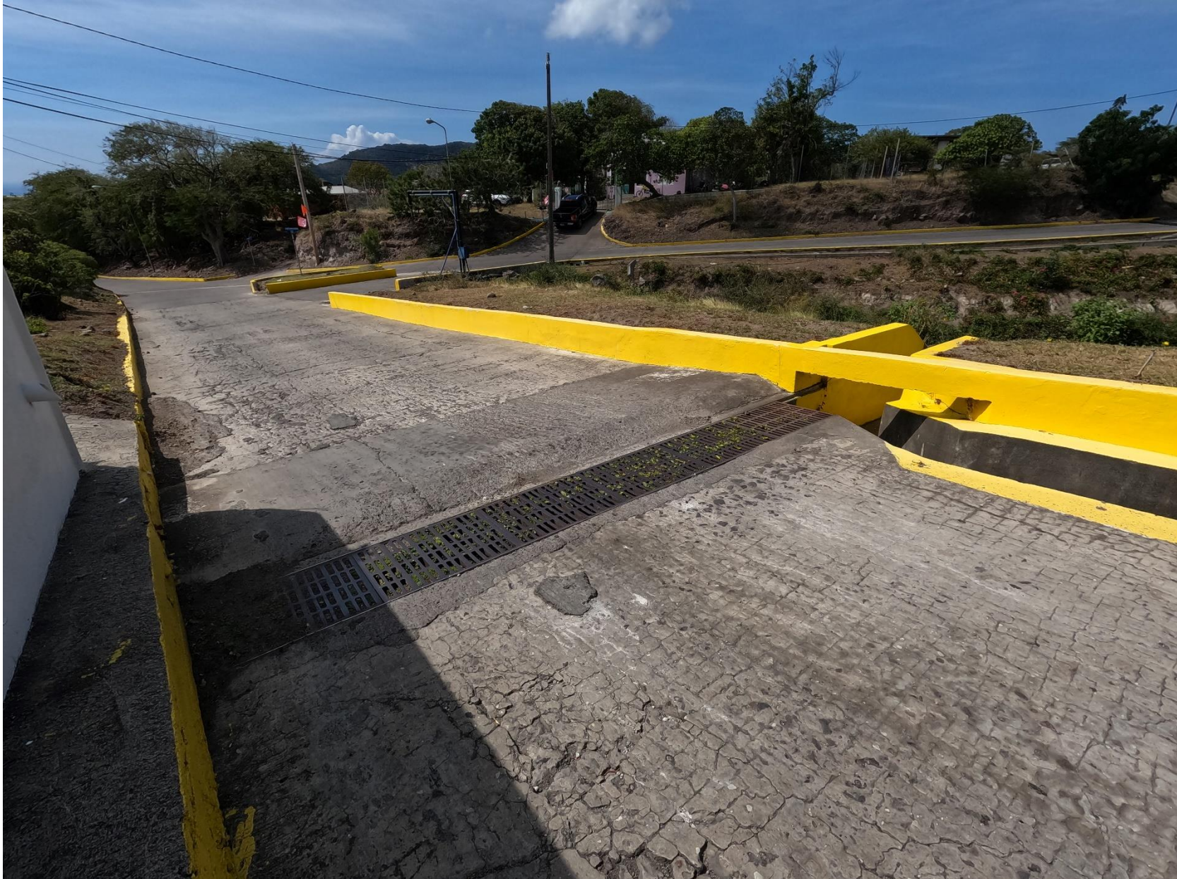
Photo 2 – Linear drain followed by a speed bump
