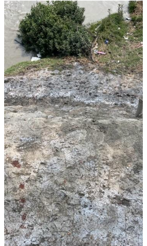
Figure 12: Salt depositions in the ground
