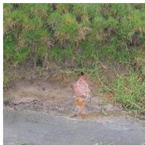
Figure 7. Iron oxidates in the drains, resulting in clogging of the drains. (Landgoed Klein Vennep, February 23, 2023).
