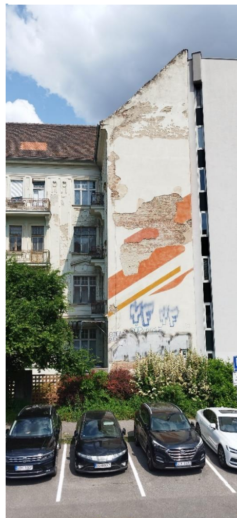
Figure 8: Deteriorating building envelope in Bratislava
