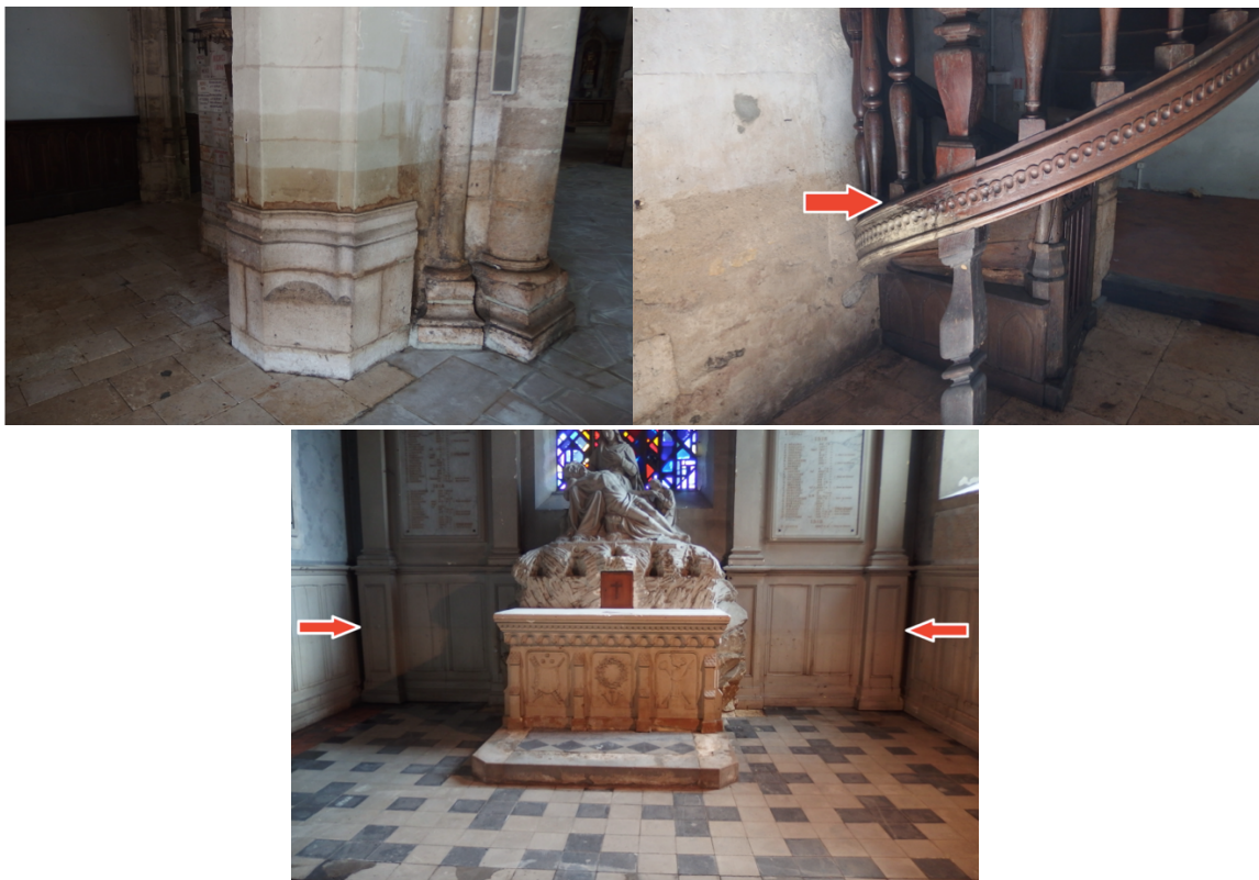
Figure 10-12 (Source: Repères de Crue): High-water marks located at + 1.13 m on a pillar of the Church (on the left) and at + 1.07 m on the pulpit (on the right), and at + 0;85m in the Chapel (down).
