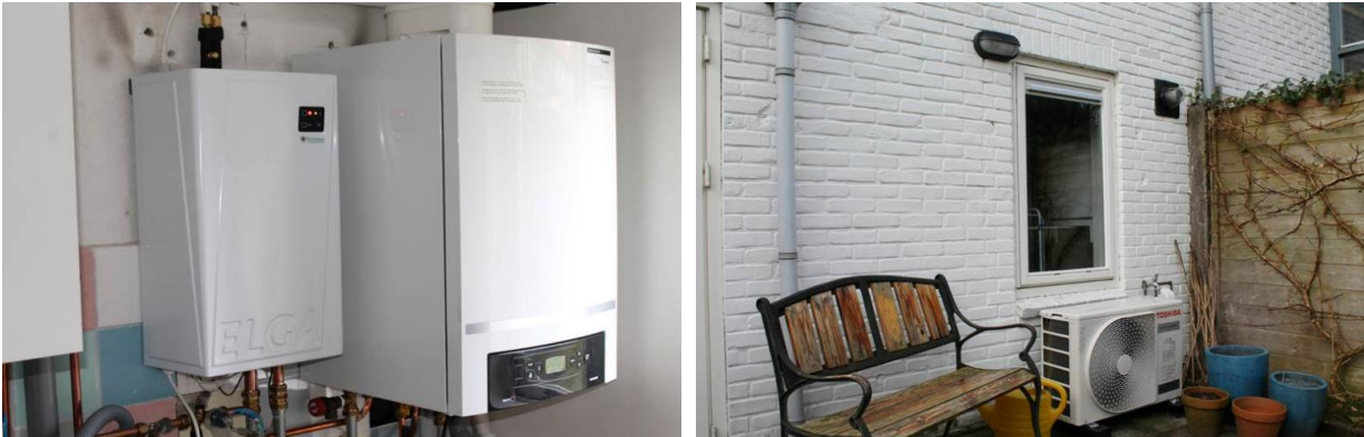
(a) Hybrid heat pump (left) with central heating boiler (right)
