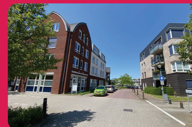
Figure 4.27: Thuvine Park in Duiven. Old nursery- and retirement homes were completely renovated and expanded.
