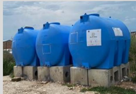
Picture 5: water tanks
