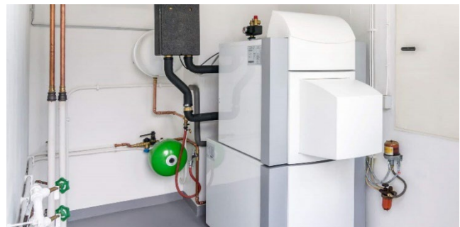
Figure 10, an installed individual heat pump.
