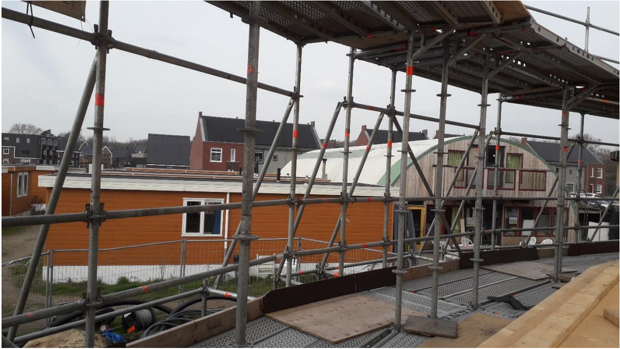
View from the third circle, under construction, on the temporary units and the Community Centre serving as common space for Ecovillage Boekel
