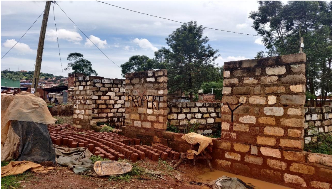
Figure 30. A typical example of an unfinished building of which further construction has been delayed by uncertainty caused by the KJE in Kasokoso.
