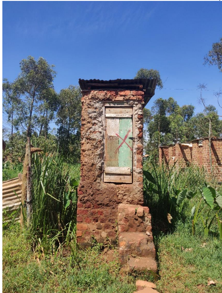
Figure 14. A toilet building marked with 'X' for removal in the KJE right of way in Kasokoso
