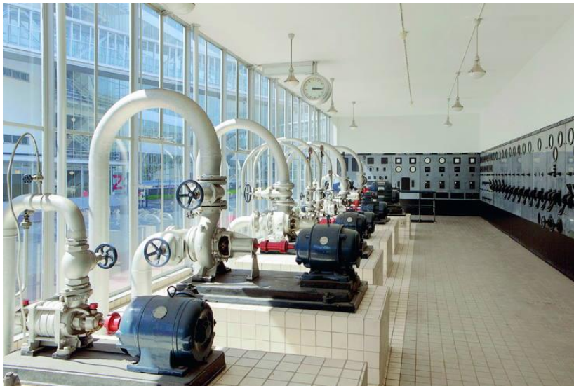
Control room in the boiler house (Aarts, 2010)
