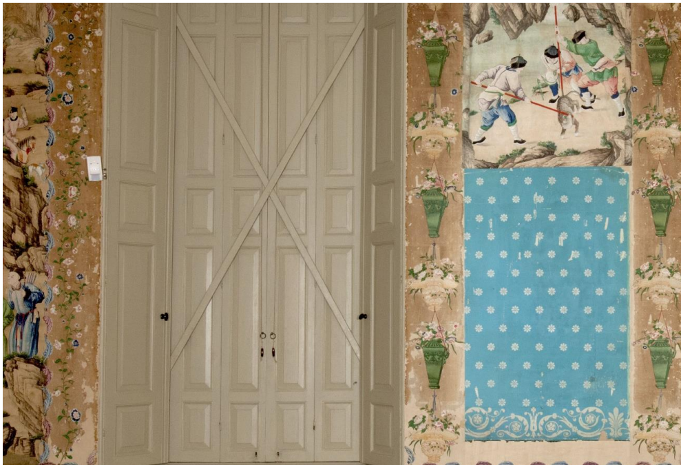
Fig. 85 - Detail of floral borders on the south-wall in Salon 1.5 at Oud-Amelisweerd. Also blue-empire wallpaper is visible, installed by Louis Napoleon © Het Utrechts Archief.
