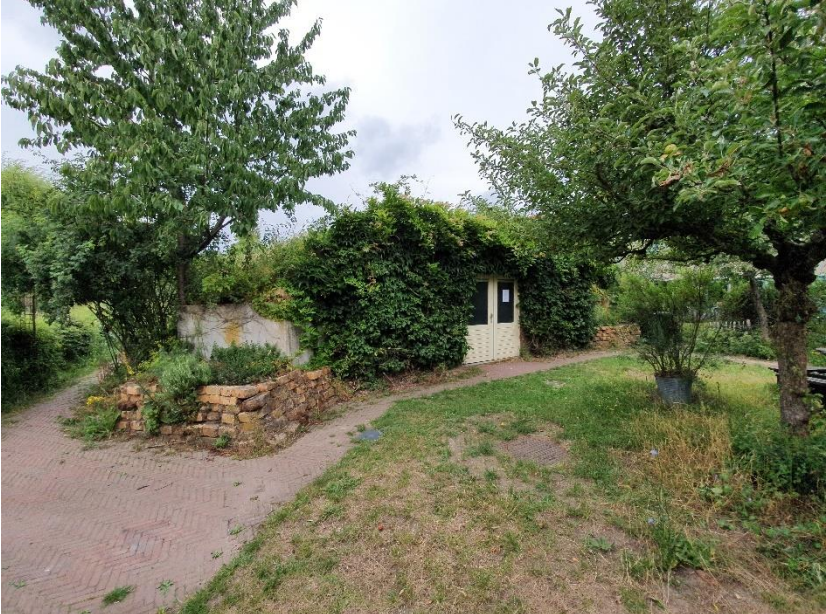
Front view of the shed where the circuit box, the control panel for the water pumps and the sediment trap are harbored.
