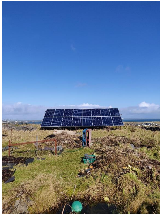
Photo 6 and 7 - Energy infrastructure at the Hill Farm: a rusty wood pellet stove on the right, and large propane gas cannisters (6), and solar panels (7) 24 February 2020
