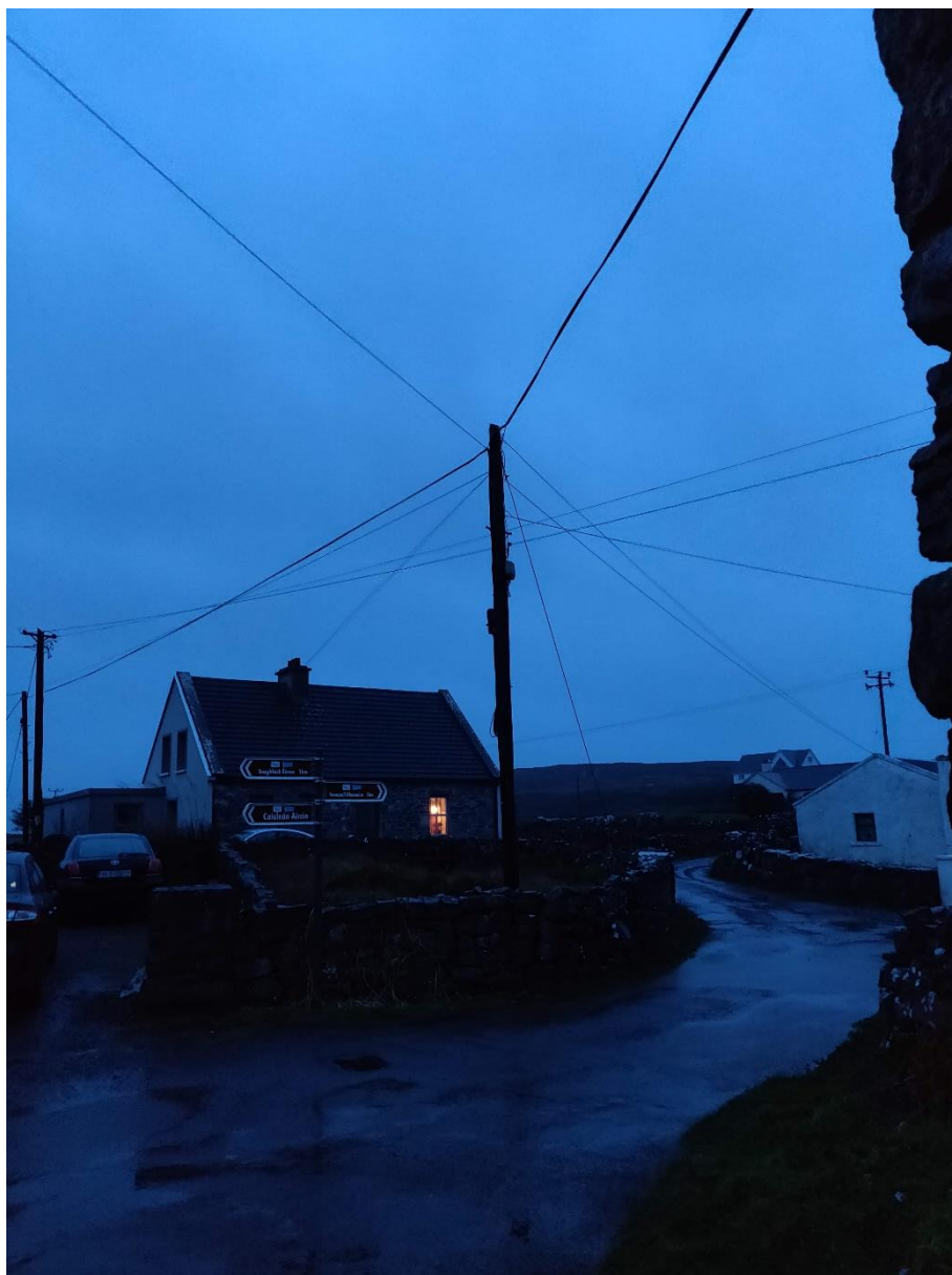
Photo 5 - Suspended electrical cables, distributing electricity to Cill Éinne homes 8 February 2020
