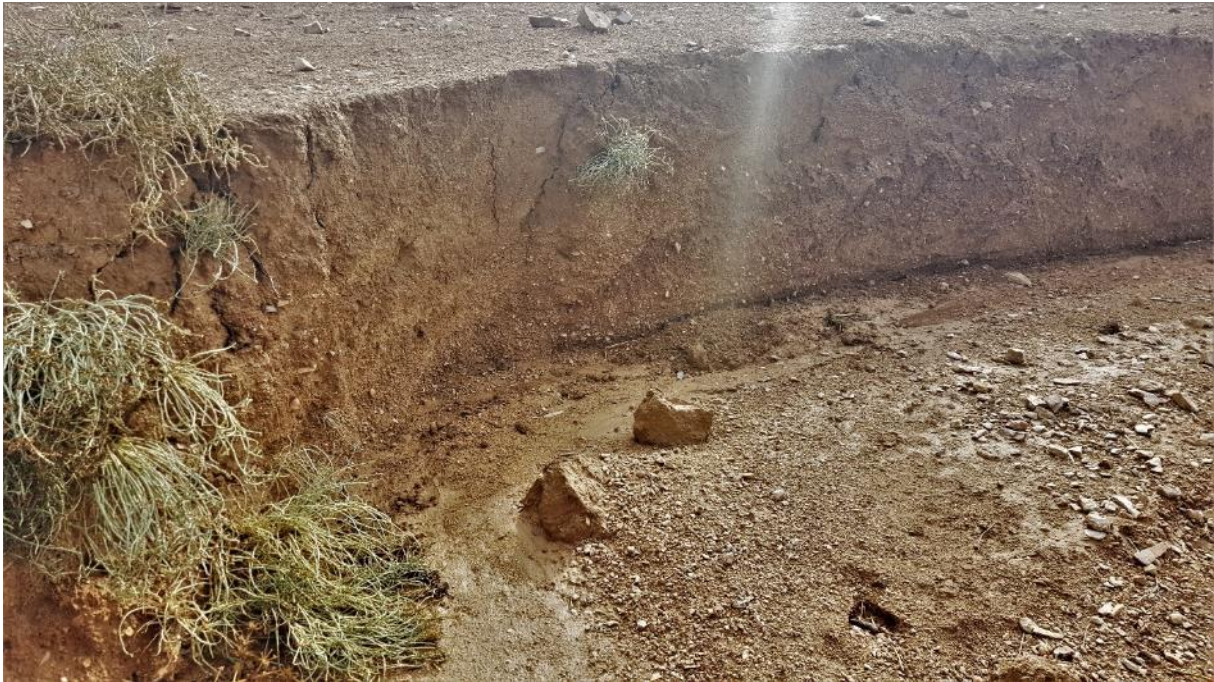
Figure 46: Soil stability and vegetation. The side wall with vegetation has collapsed due to erosional forces exceeding the stability forces.
