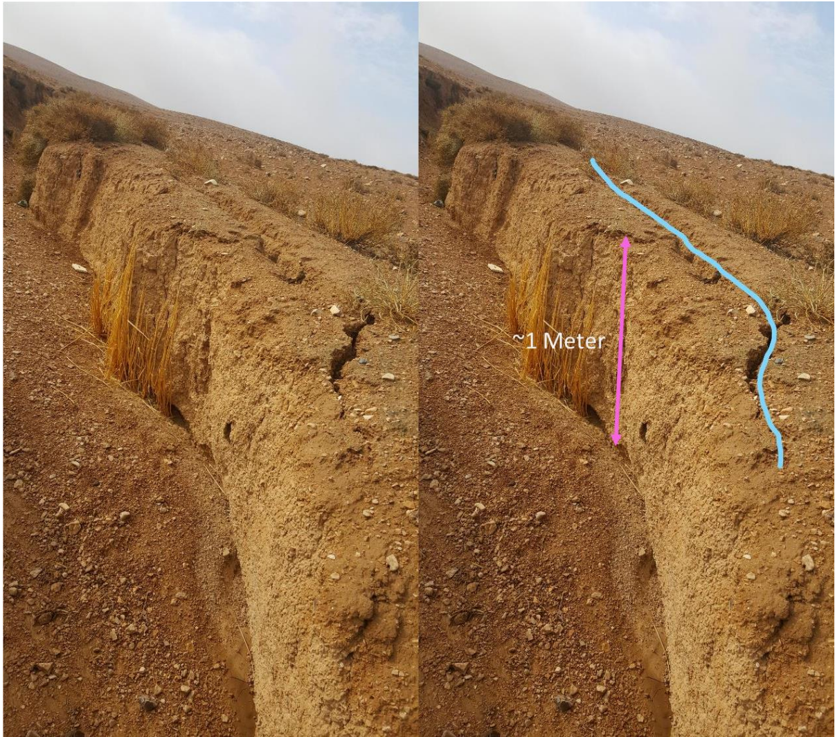
Figure 37: Spliced earth as seen in the gully (blue line). The side bank can collapse after undermining by scouring.
