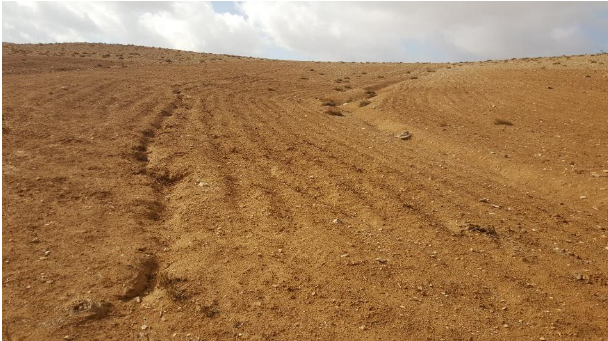
Figure 47: Forming of rill erosion by contour plowing parallel to a gully tributary.
