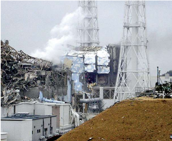
Figure 5. Destruction at reactor 3 of Fukushima-Daiichi power station, March 15, 2011.
