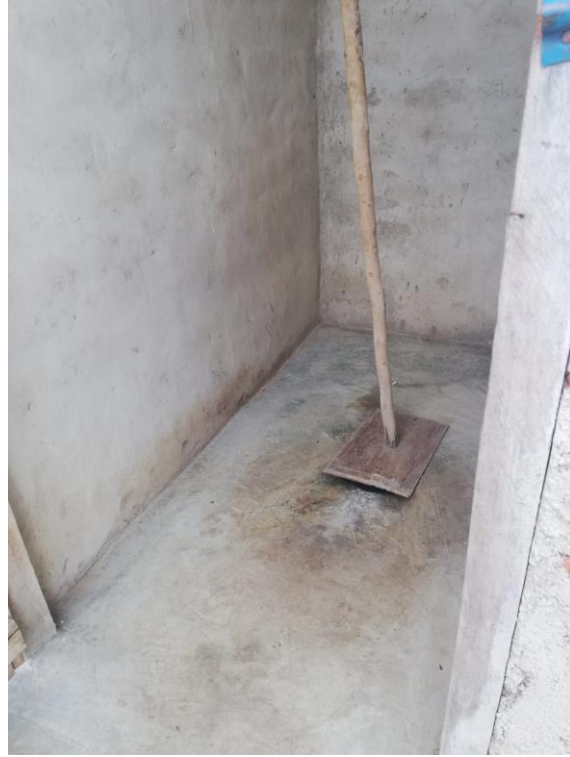
Photo 6 - Latrine where lid cover deemed improper. Author's own.
