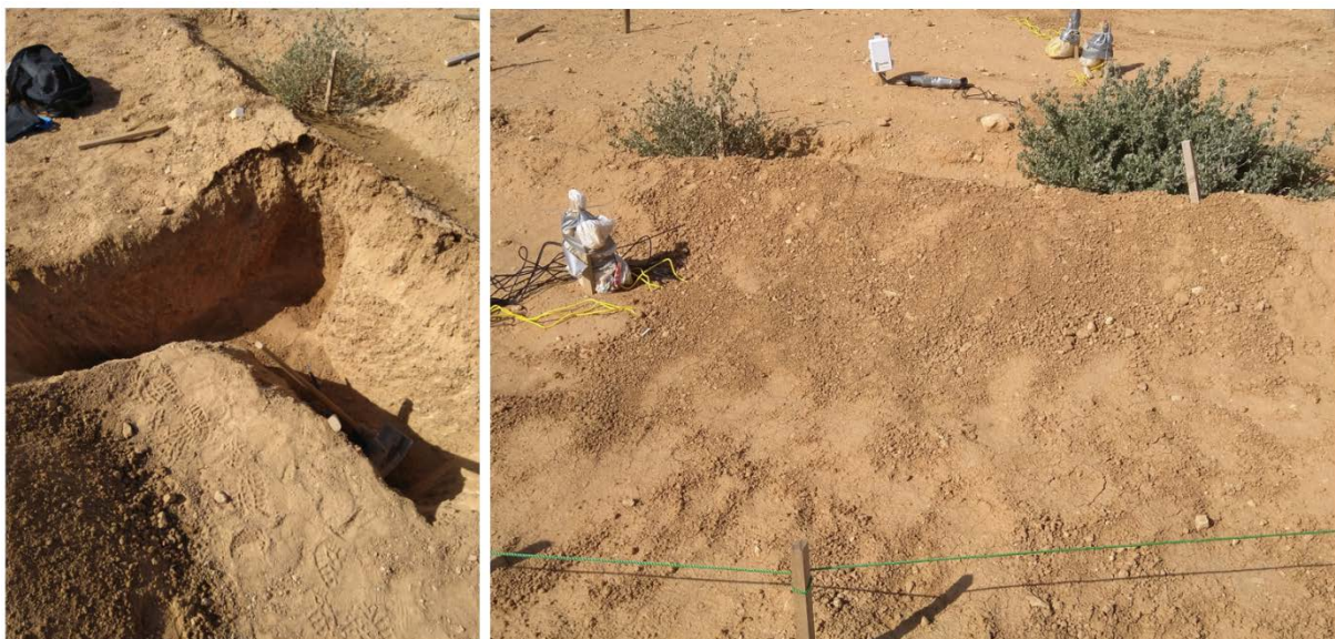
Figure 10 Left: Picture of the cut used to install the Decagon 5TE sensors. Right: The Vallerani RWH structure after the cut was filled up.
