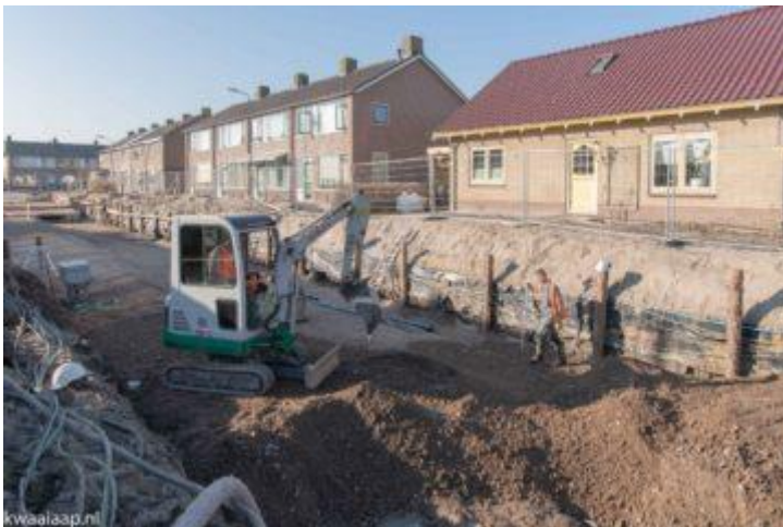
Image 7: The scope and length of the construction makes this a tricky project. Source: Author
