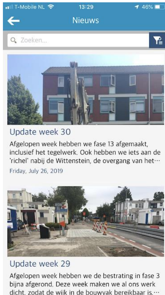
Image 5: The Update screen of the Omgevingsapp reconstruction Assumburg. The weekly updates contain pictures that show what the contractor has been doing for the last week.
