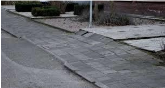
Image 6: The unsolid ground under de Kanis is causing visible damages to the infrastructure and foundation of the village. Source: Stakeholder Manager
