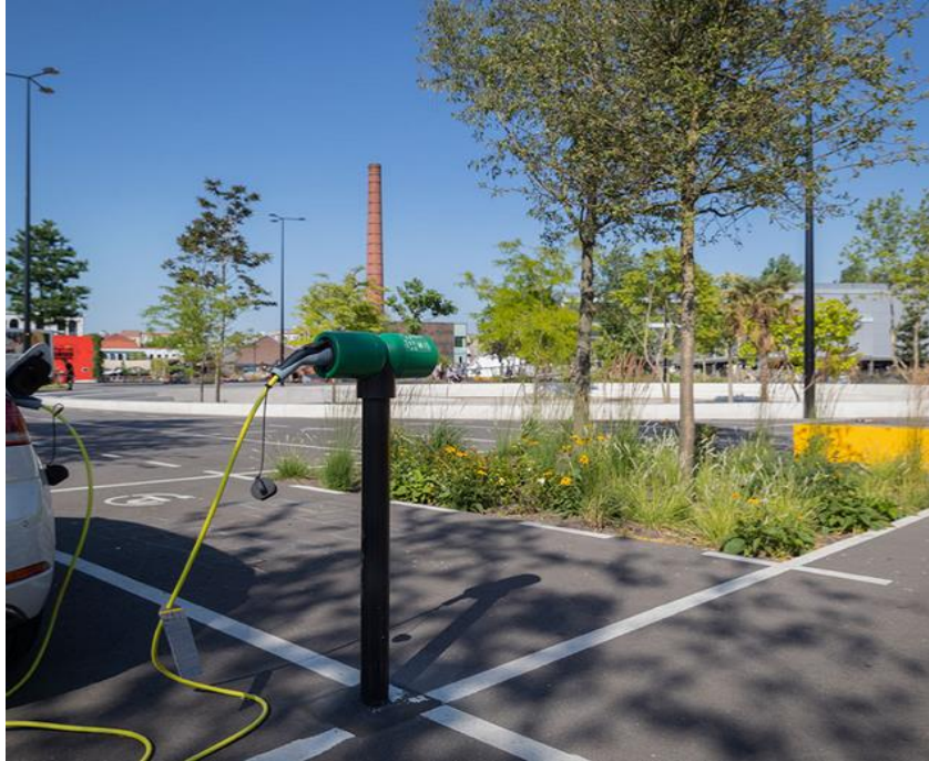
Figure 24 Example of an electric charging pole on the square. Source: VIC Activating Landscapes (n.d).
