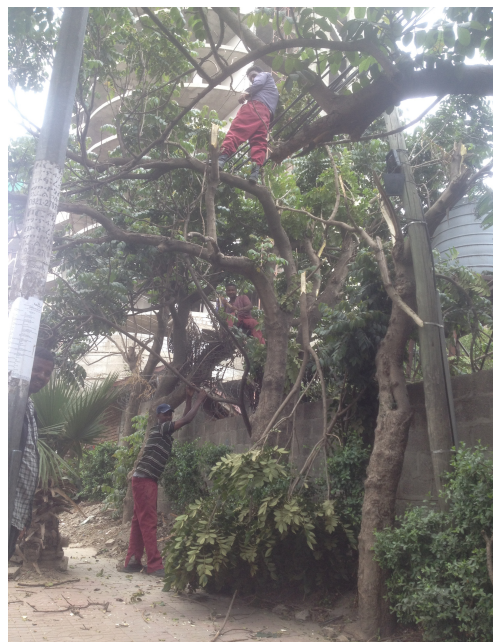
figure 3.2 - Workers in the City area of Addis Ababa, trimming branches of trees close to high intensity electricity. As one can not they were not working under the necessary safety measures. This is a testimony of the high degree of informality of Ethiopian everyday economy.
