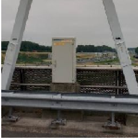
(b) Image of a cabinet house
