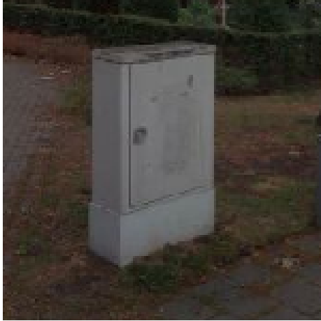
(a) Image of a CAI cabinet
