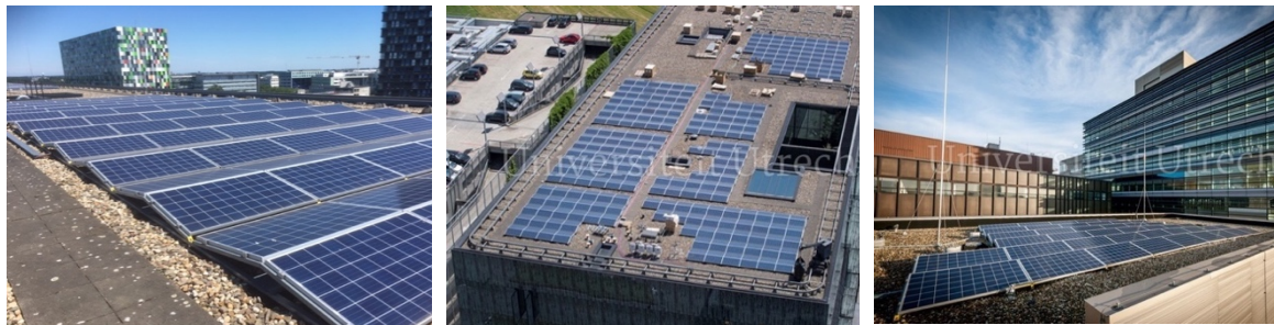
Figure 4. Rooftop PV in the Uithof (Source: Utrecht University)
