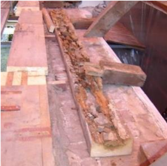
Figure 9 - Wood decay in wall plate caused by fungus
