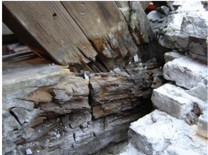
Figure 10 - Wood decay in load bearing beams in the roof construction caused by fungus
