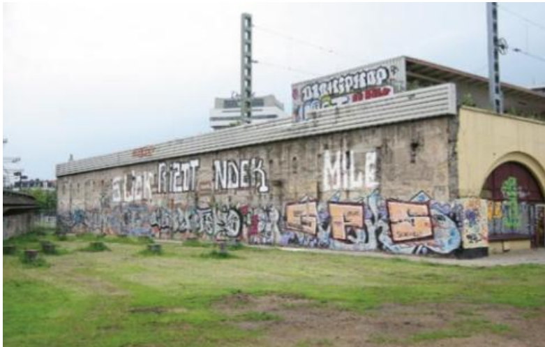
Image 4.1: The decay of Station Hofplein and the 2 kilometres of railway viaduct in Rotterdam set in since the station was abandoned and closed, resulting in vandalism. Nevertheless, the station and viaduct received a monumental status in 2002.
