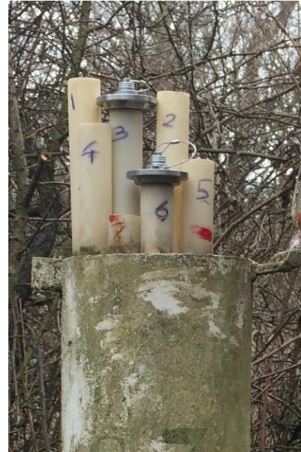
Figure 12, Monitoring well B2F0072 with three ADCs installed for screen number 3, 6 and 9 (screen 9 is below the monitoring well mantle)
