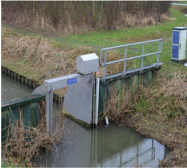
Figure 8 Dynamic weir (department RA, 2019)
