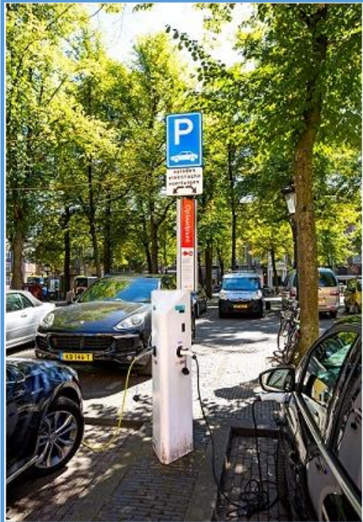
Figure 5: Example of a charger. A charger is placed in public space with two reserved parking spots and enables two electric cars to recharge their batteries simultaneously (PitPoint image bank, 2018).
