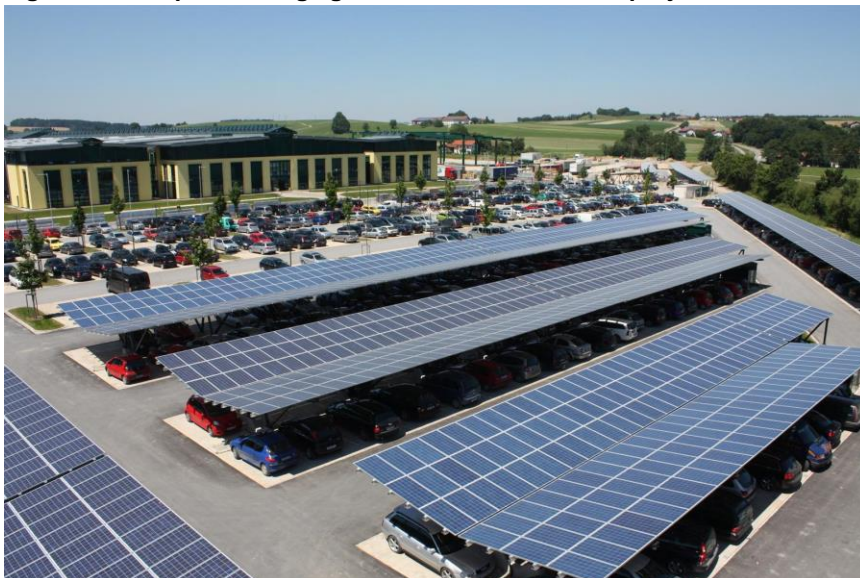
Figure 2. Example of a large ground mounted solar PV project combined with mobility.
