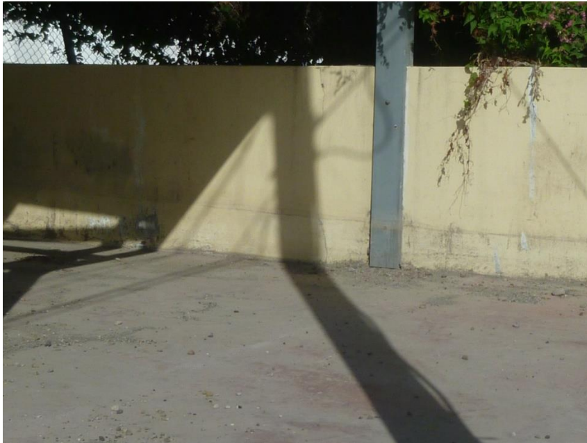
Figure 5.9: Mud marks on the wall of an old petrol station in the harbour area. Mud marks originate from a landslide that happened in November 2016. Marks reached up to a meter high.
