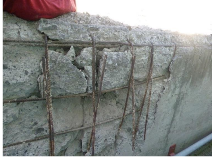
Figure 5.12: Metal of reinforced concrete bent by a boulder that fell from the cliffs in the harbour area.
