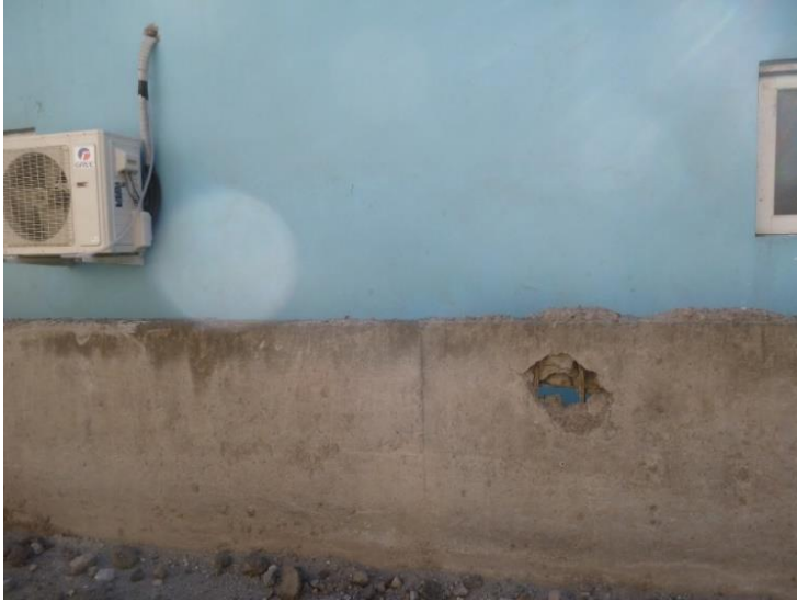
Figure 5.11: Small wall in the harbour area with a hole created by a boulder that fell from the cliffs.
