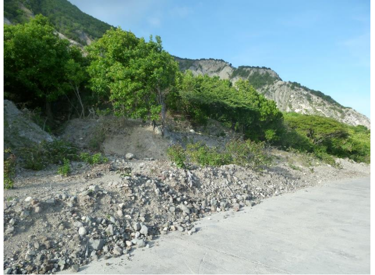
Figure 5.7: Left-overs from a recent landslide that occurred in November 2016 and covered the entire road.
