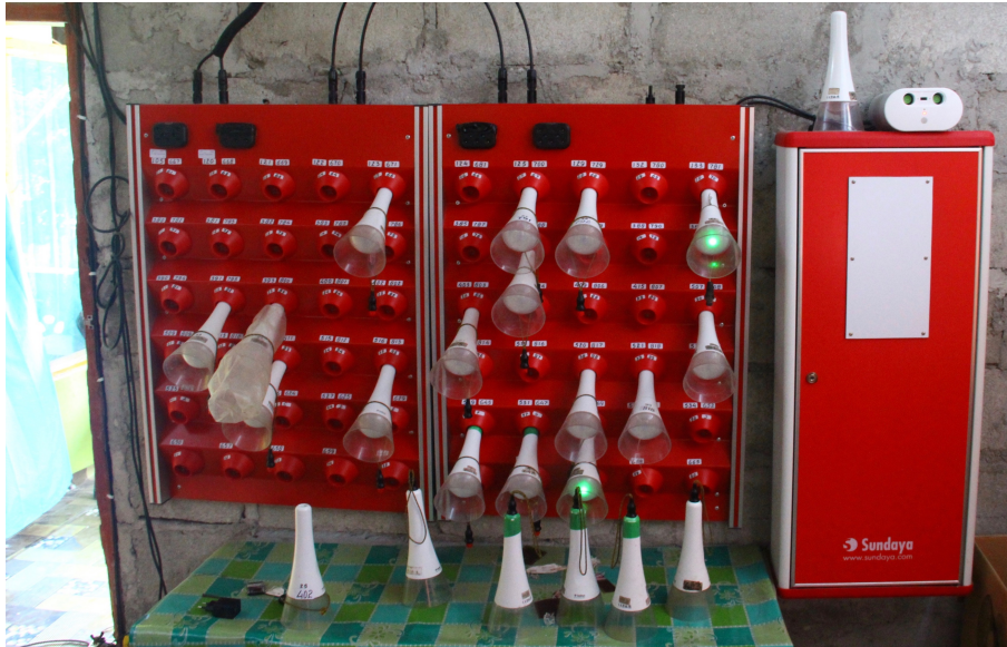
The charging board for the lanterns.
