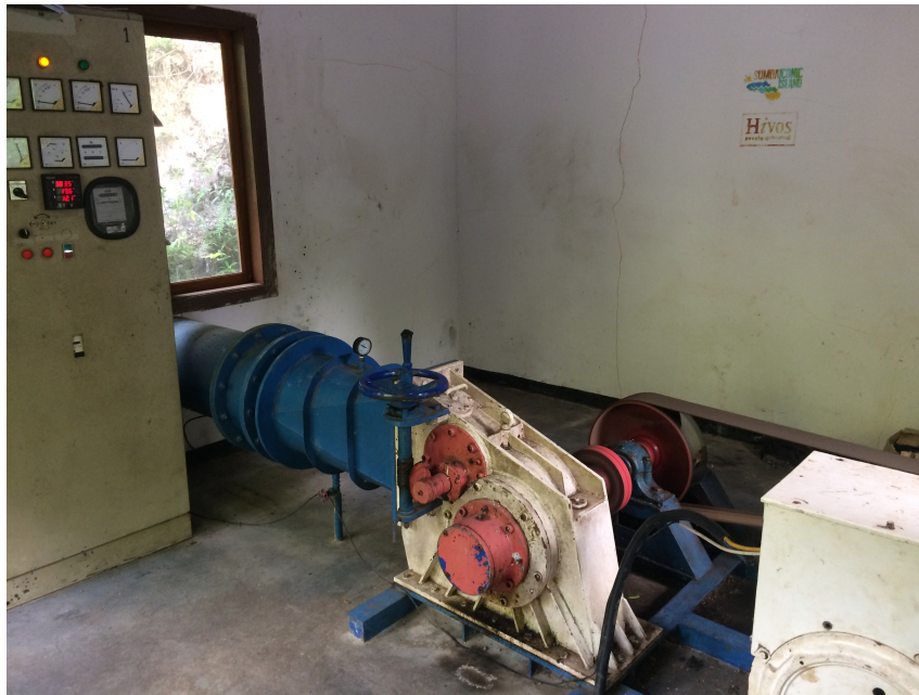
One of the micro-hydro installations.
