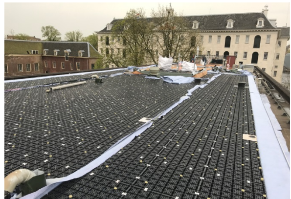
Figure A2 Placement of the permavoid units during construction of the green roof.
