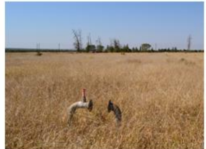
Photo 2 Disconnected irrigation pipe in Giyani (Fröbrich, 2014)
