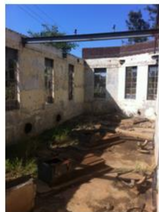
Photo 3 Broken water pump house in Giyani (own photo)
