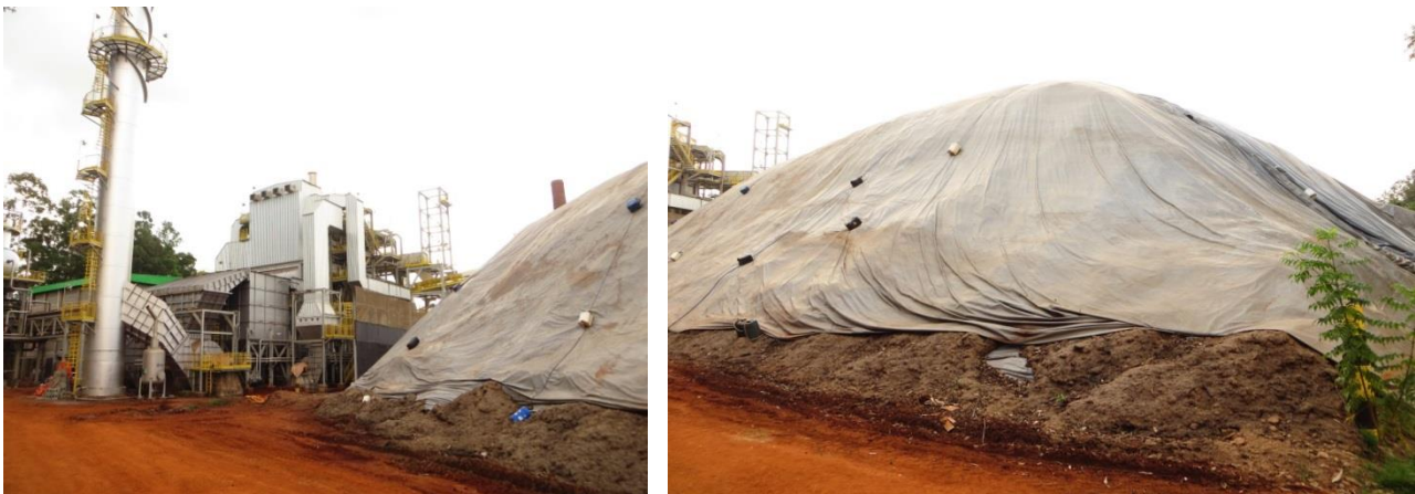
Figure 18 Left: steam boiler for firing bagasse. Right: stored leftover bagasse from previous season. Araras, São Paulo (own photos)
