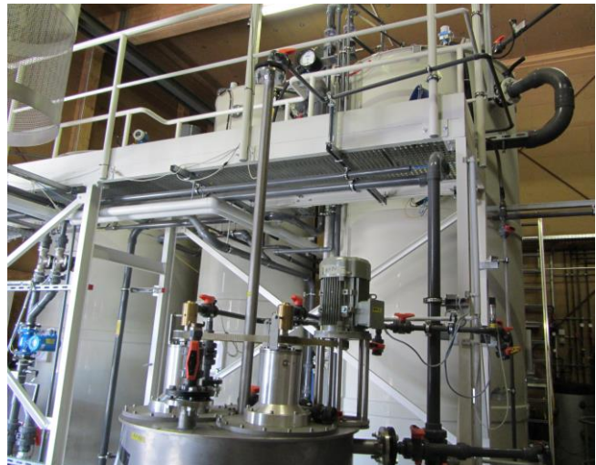
Figure 4.11 The anaerobic MBR for biogas production
