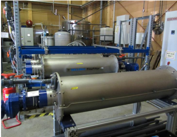
Figure 4.12 The water filters for upgrade of wastewater to service water
