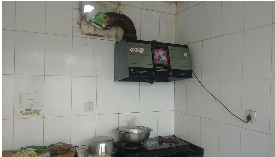
Figure 9. Structural adjustments to adapt the kitchen to improved electric cookstoves, new Simatai village. July 23, 2017.
