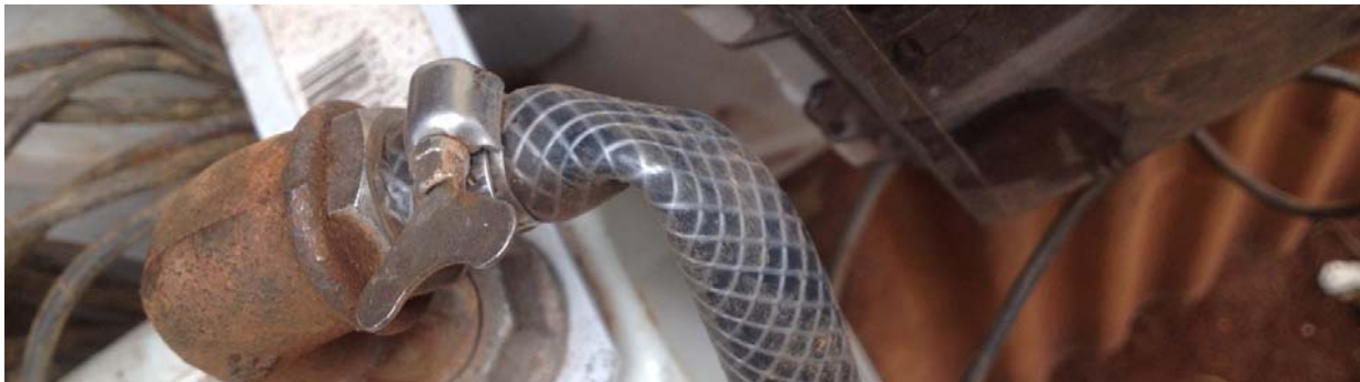
Figure A 7: picture showing kinking of the hoses that are used to connect the data logger with the biodigester piping. Picture from own archive.
