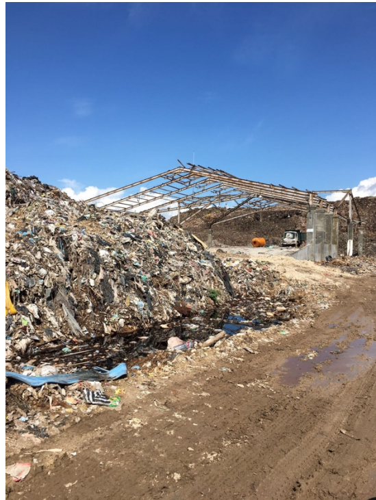
Figure 19: The demolished Galfad plant of NOEI.
