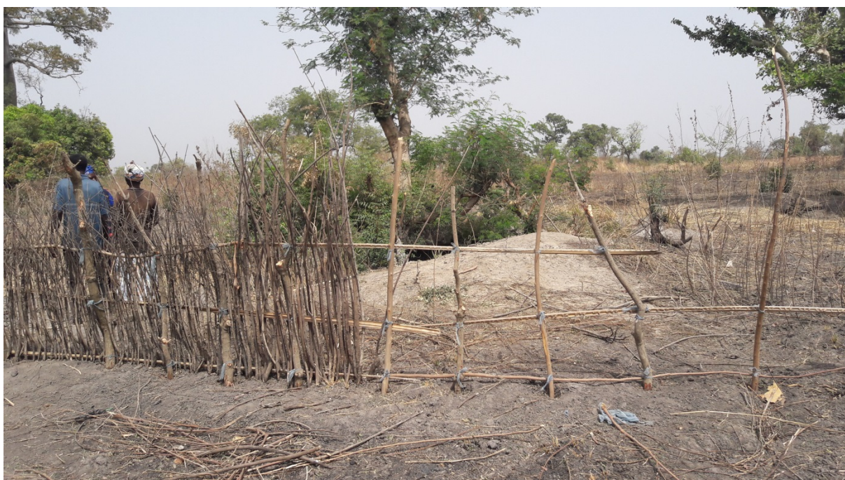
Figure 8. In the foreground, sticks fence under construction. Picture taken by the author.
