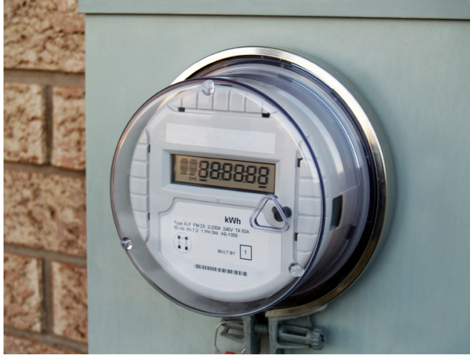
Figure 2: The smart meter comprises of a computer and a sensor for measuring electrical consumption.
