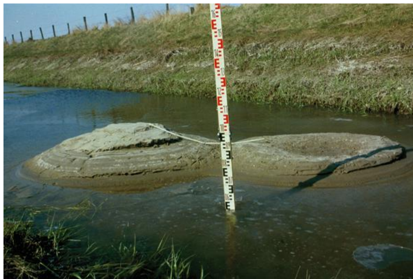
Figure 1.3 Two observed boils near a dike, with sand eroded from the aquifer towards the surface [https://beeldbank.rws.nl, Rijkswaterstaat].
