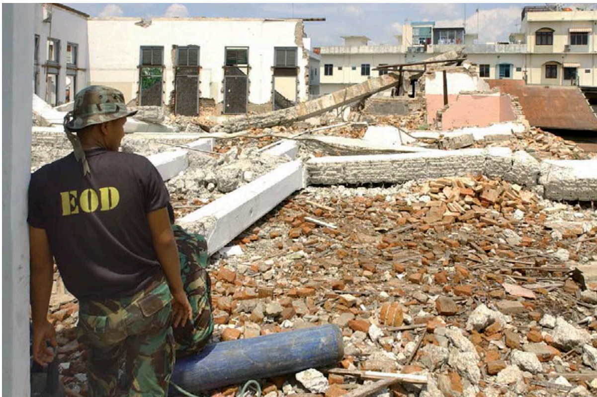
Fig. 4.6. Despite public protests and despite police supervision, demolition of a Dutch colonial factory in 2002 could not be restrained.
