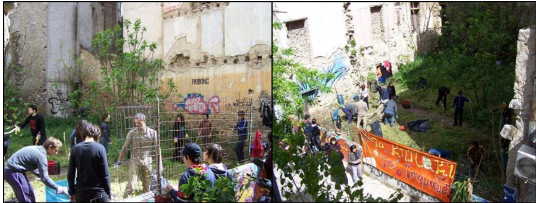
Picture 19,20. The work in progress at the vacant plot in Tsamadou Str. Source: https://athens.indymedia.org/post/849170/
