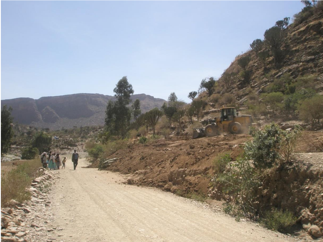
Figure 5 – Sub-road construction in progress in the research village Adikisandid. This sub-road will allow big trucks to reach stone-grinding facilities. Meanwhile a group of women passes by as they are walking along the existing main road through the village.
