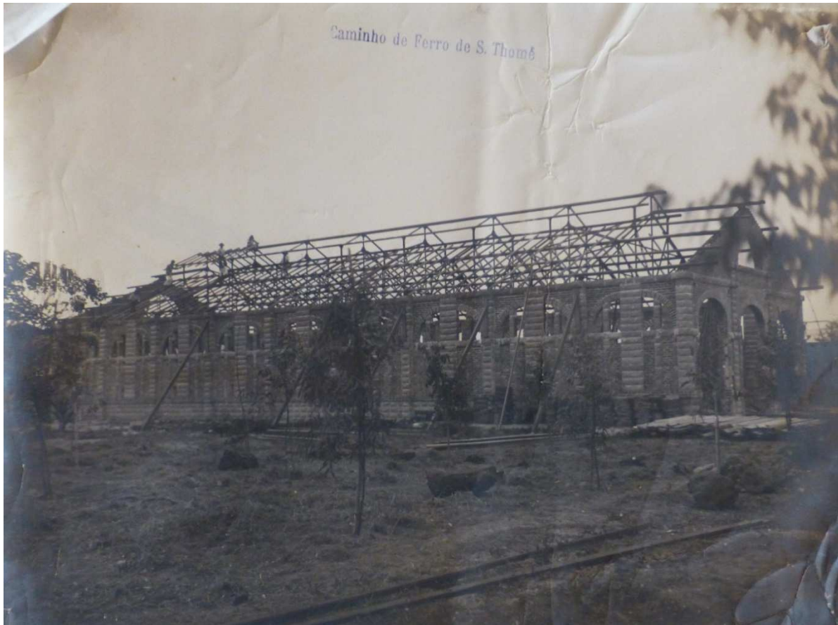
Fig. 60. Exterior train shed of the S. Sebastião Maritime Station during construction in 1910, providing a rare view of how these buildings were put together.
