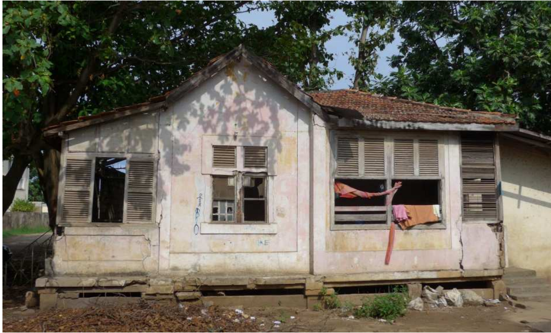
Figs. 97 and 98. Facade and long side of the guard's cottage at the S. Sebastião Maritime Station, 2015.
