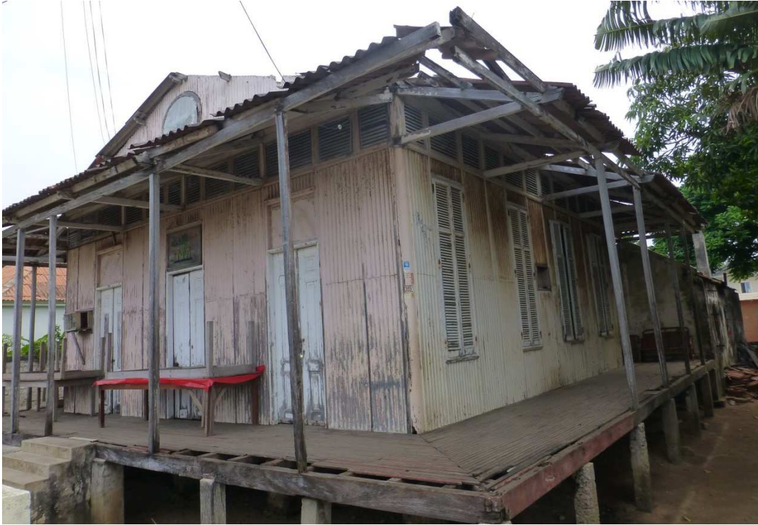
Fig 111. Facade and side view of one of the four sea fronting workers cottages, in ruins, 2015.
