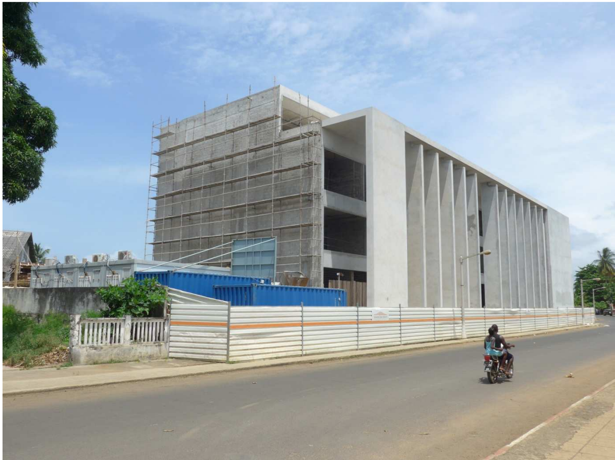
Fig. 108. Central Bank of São Tomé under construction - general view, 2016. Part of the roof from the former railway workshop ( Cacau ) is visible on the left.
