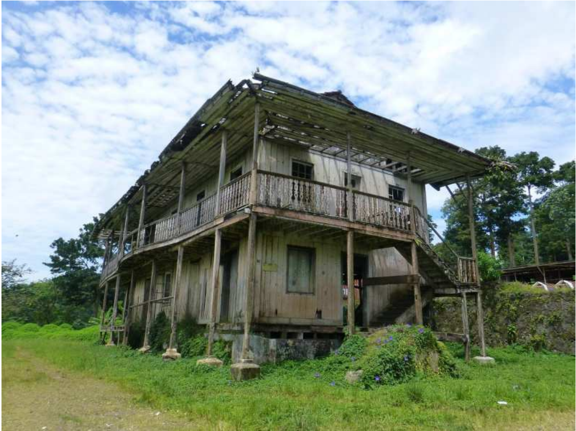
Fig. 30. Roça Nova Moca's main plantation house, close to collapsing, 2014.
