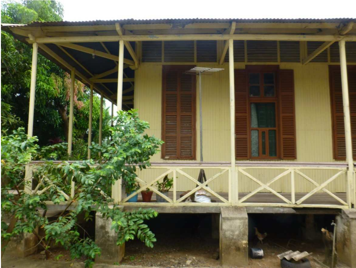
Fig. 91. Long side of the 5th workers cottage, adjacent to the S. Sebastião station building; note the elevation, louvered windows and transoms as typical features of architecture for the tropics, 2015.
