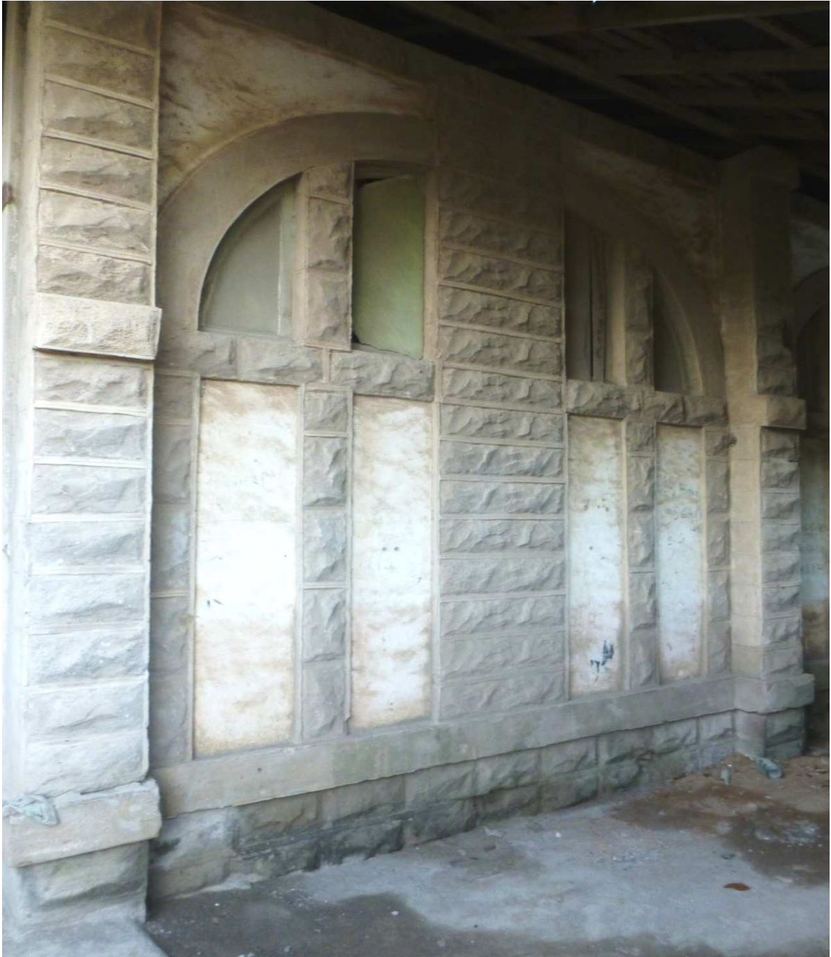
Fig. 65. Train shed at the S. Sebastião Maritime Station, detail of a semicircular arcade, 2014.
